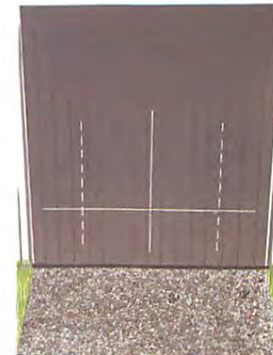
Measure the height of the lamp centres from the ground. Draw a horizontal line on the wall at this level across the vertical lines already in position.
