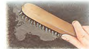
Remove loose sealant and clean the spot with a stiff wire brush.
